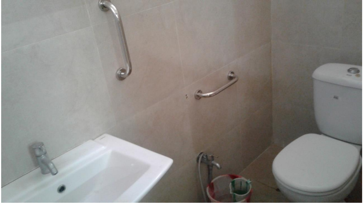
Figure 3: Toilet for handicapped students
