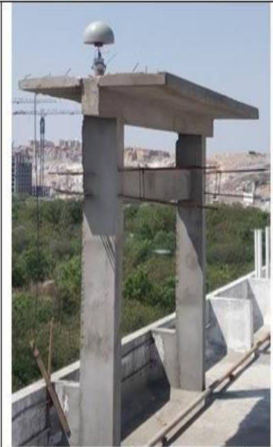
Fig.2 Antenna Mounted at rooftop of R&E Hub
